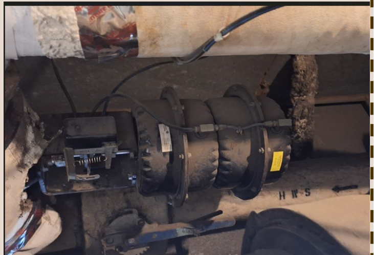
Example of “existing” pneumatic equipment to be replaced .
